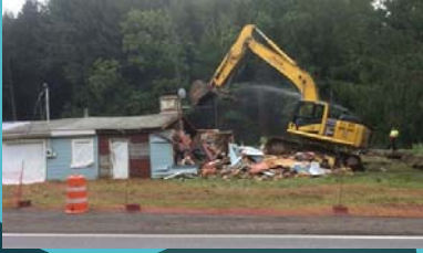
CWC funded demolition of home along Manorkill Stream in Town of Conesville
