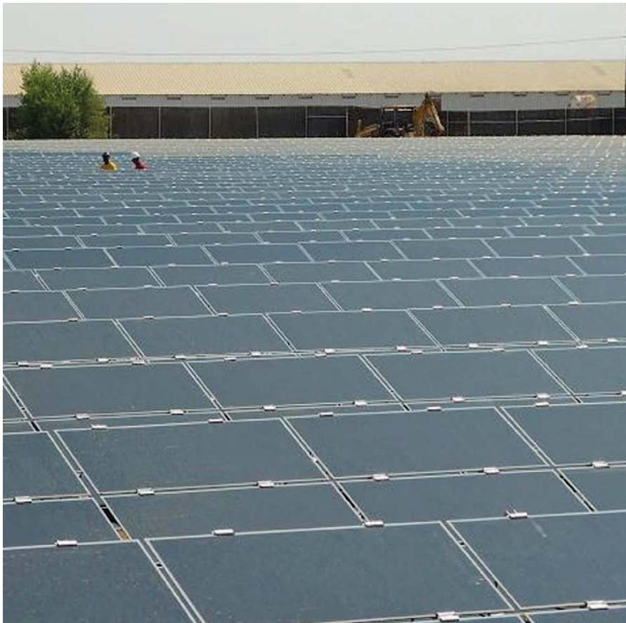
Photo from SMUD's SolarShares Installation
