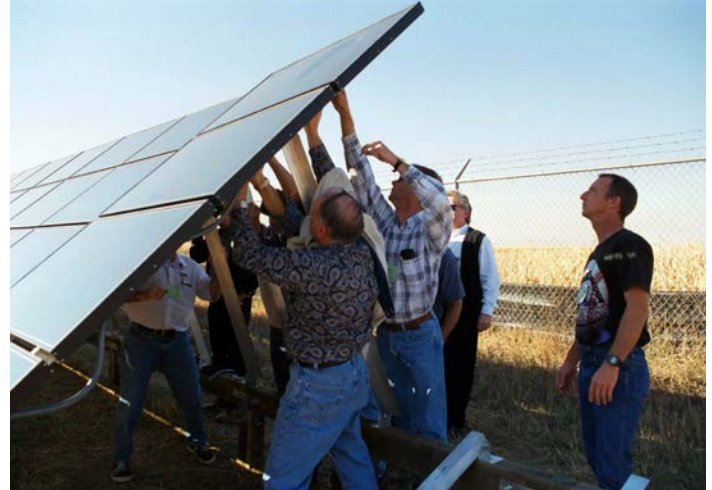
Photo by Western Area Power Administration, NREL 08822
