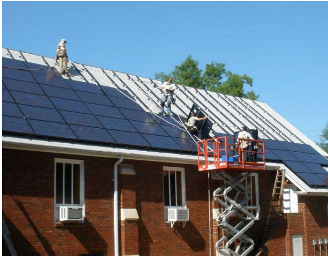
Photo from David Brosch, University Park Community Solar, LLC
