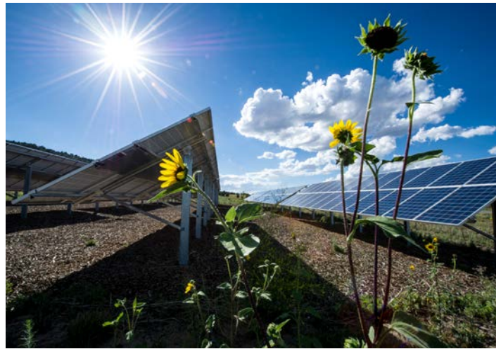
Photo by Dennis Schroeder, NREL 26962
