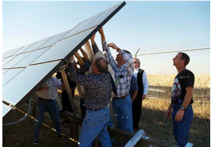
Photo by Western Area Power Administration, NREL 08822
